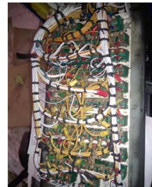
The completed circuit breaker panel, looking a lot tidier than the one it replaced.
