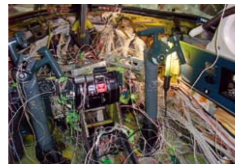
With panel removed, work began to also remove a great amount of redundant wiring.
